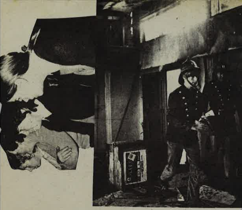
Firemen work their way through the smoky haze after flames engulfed a section of the new classroom block currently under construction at the Tokoroa High School. The cause of the fire, which occurred on Saturday, is not known. — Story page 3.
